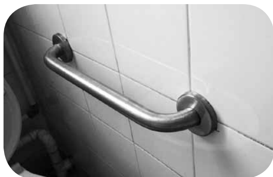
現時為長者戶安裝在洗手間內的單枝扶手。 This is how a grab handrail looks — a grab handrail installed in toilets for elderly.
