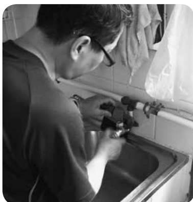
義工師傅正協助徐婆婆更換水龍頭。 Volunteer technician is helping to replace the tap for Granny Chui.
