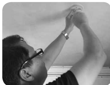
義工師傅正協助簡婆婆拆掉舊燈座及更換新燈座，以改善照明。 Volunteer technician removed the old light socket and then replaced a new one so as to improve the lighting for Granny Kan.
