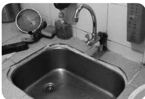
更換了水龍頭後，周伯伯不用再擔心長期漏水的問題。 Installation of a new-fashioned water tap has solved the problem of water leakage for Grandpa Chow.
